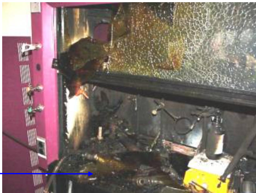
Photo 3. Fume hood after the fire. The arrow indicates the location of pipettes and cleaning wipes left by the researcher.
